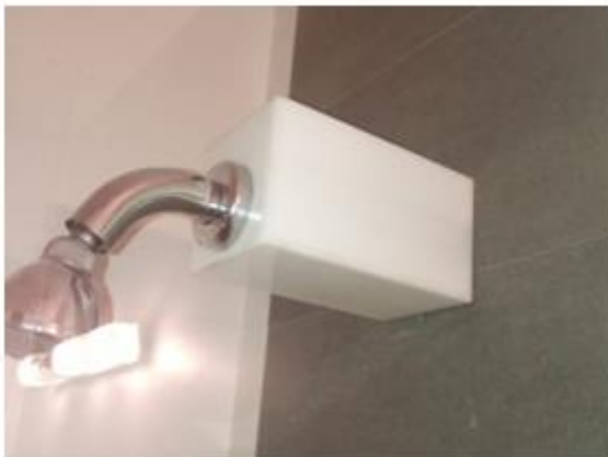
Figure C3: Example of a flow meter cover around the pipe behind each shower-head
